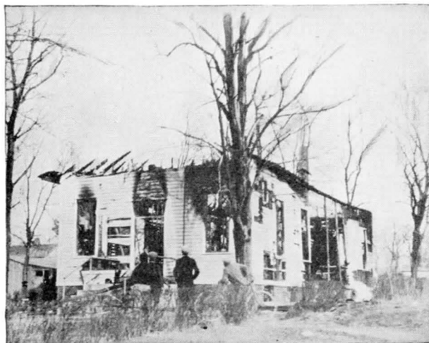
16. Ruins of colored school building, Red Bank, N. J., set fire by whites as a sequel to race war at Carteret, N. J.
