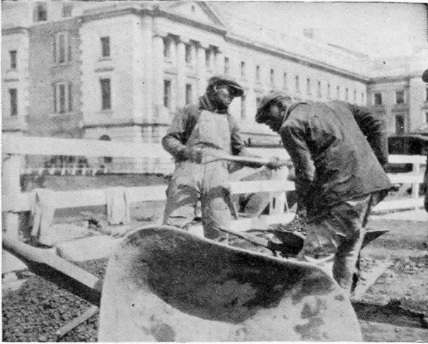
3. A large amount of construction work in Washington is performed by Negroes.
