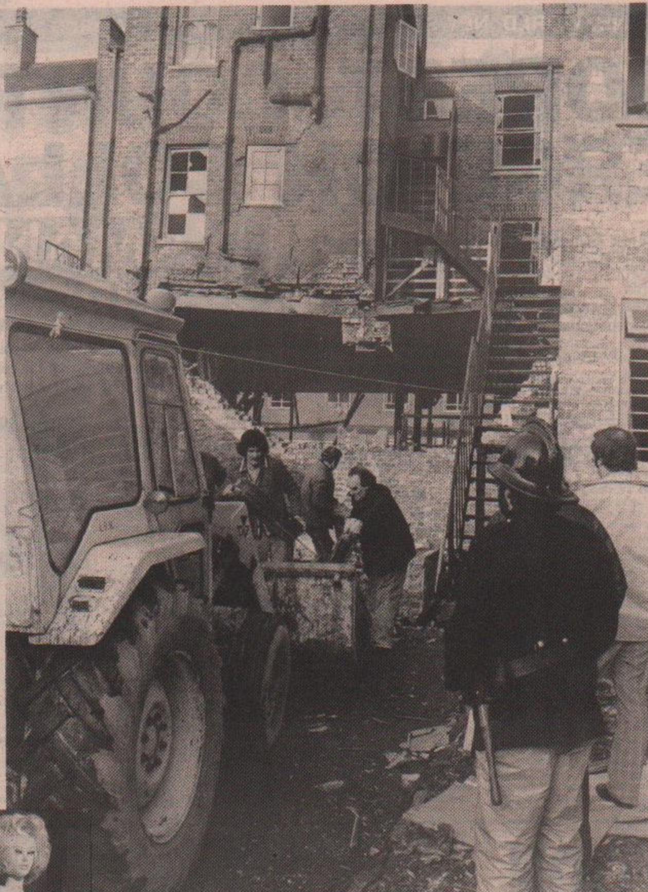
The upper storeys of the blasted shop sag and walls crack as cleaning up begins in Brentford
