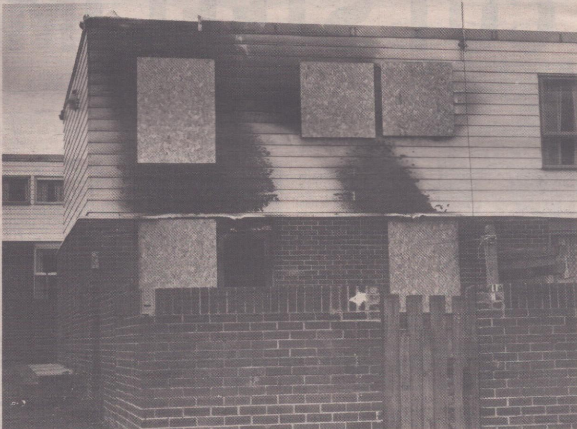
Boarded up, burnt-out houses are becoming a familiar sight in Winsford. In this case a child died
