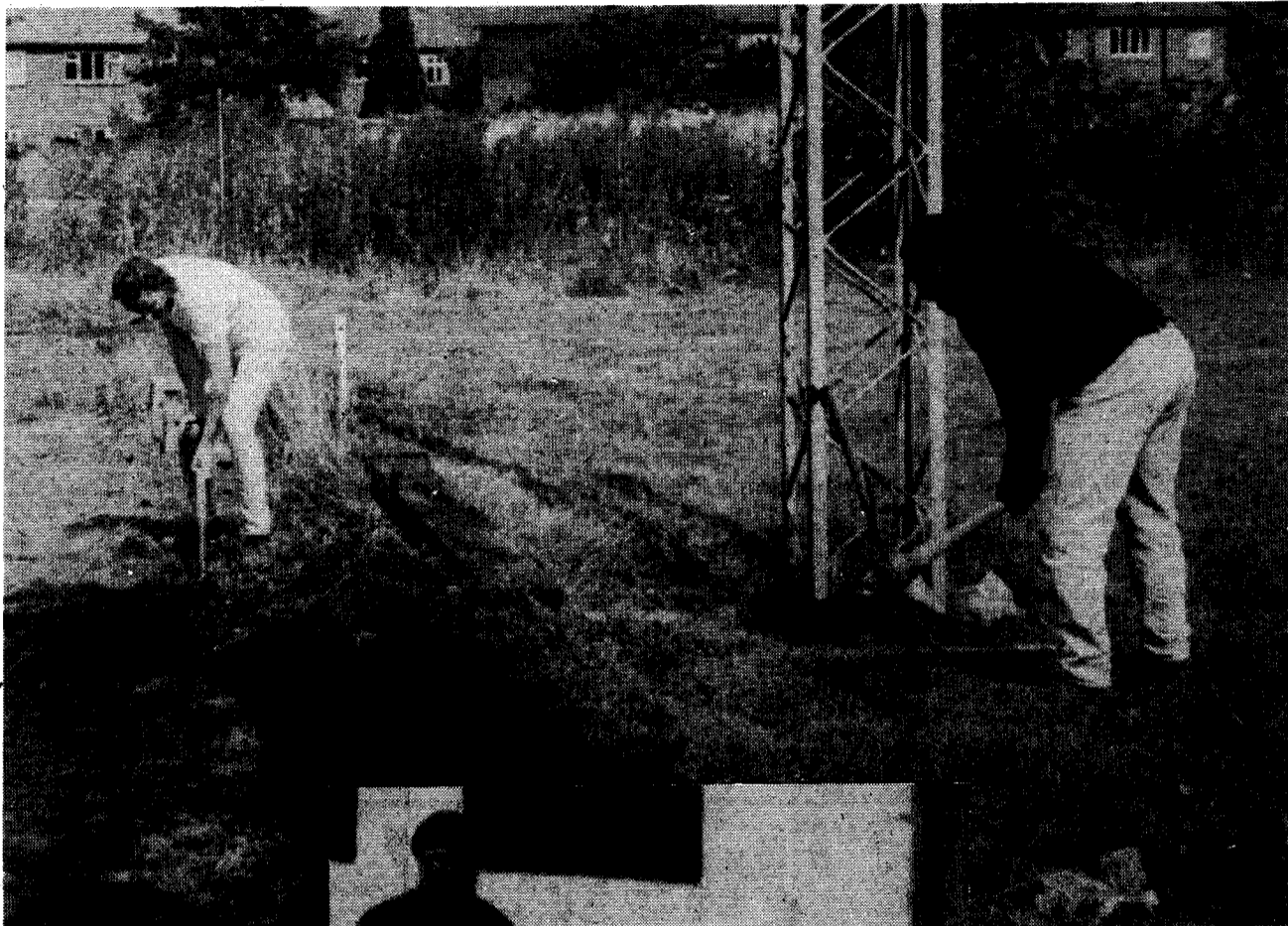
'We are supposed to be doing construction work but all we do is to stand in the middle of a pond and shift muck'
