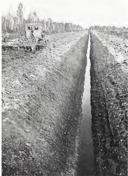
Extensive land reclamation is going on in the Estonian Republic. Here we see a deep drainage channel in previously-boggy land, which is now fit to plough.
