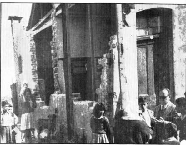
JOHANNESBURG: Four-year-old Abbot Ebrahim narrowly escaped serious injury when workmen started demolishing the walls of the room in which he was still sleeping. As a result of this demolition, the Ebra- him family had to abandon their home and move in with a relation. The landlord claims he received an order from the City Engineer to demolish and rebuild the wall of the property facing the lane. He had strted on the demolition when his tenants, Mr. and Mrs. Ebrahim and their five children, got a court order restraining him. "How can demolitions start when people are living in a house?" they demanded.
