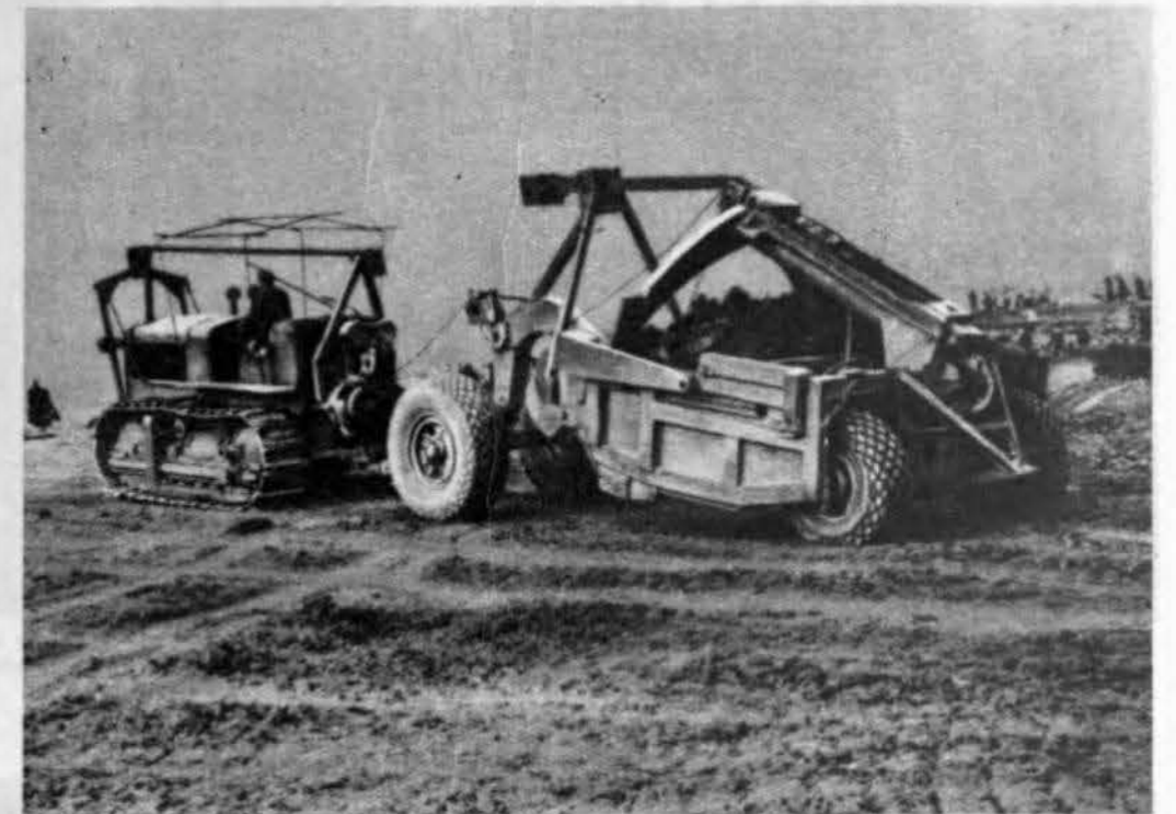
One of the many excavators at work on the sites of the dams
