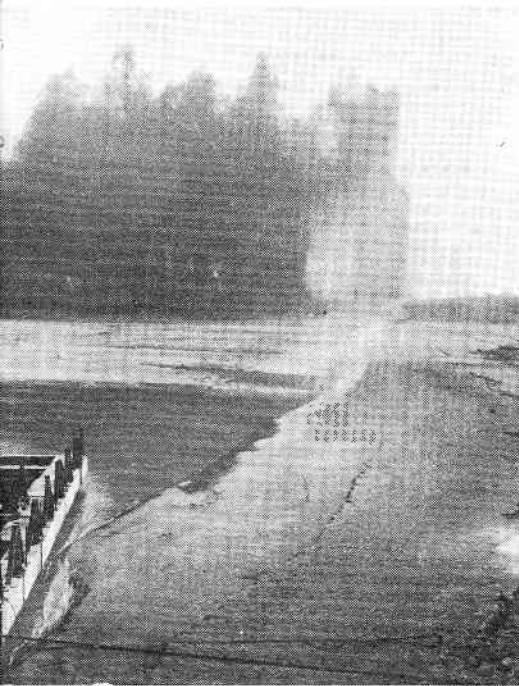
Dynamiting the bed of the Yellow River before laying a pipeline across it. Hsinhua
